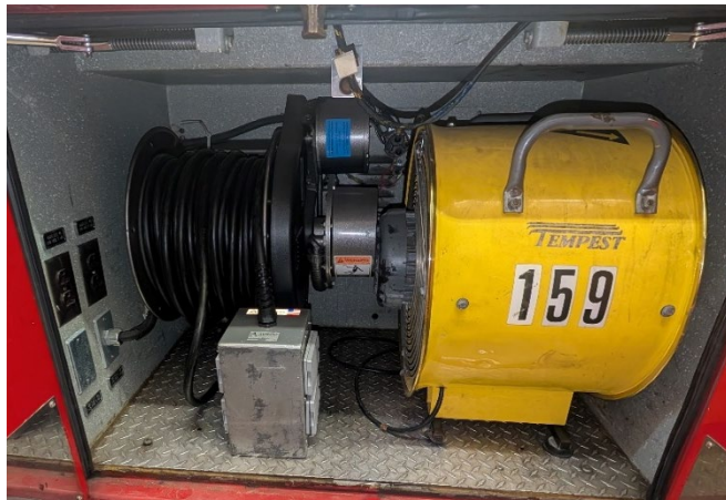
The equipment is old and obsolete.
