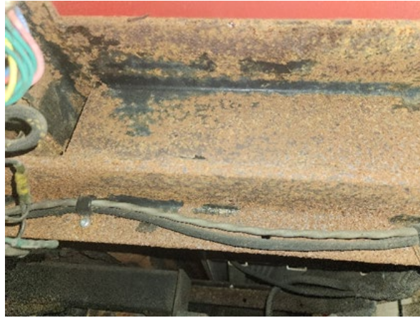
Surface rust on the underside of Engine 161.
