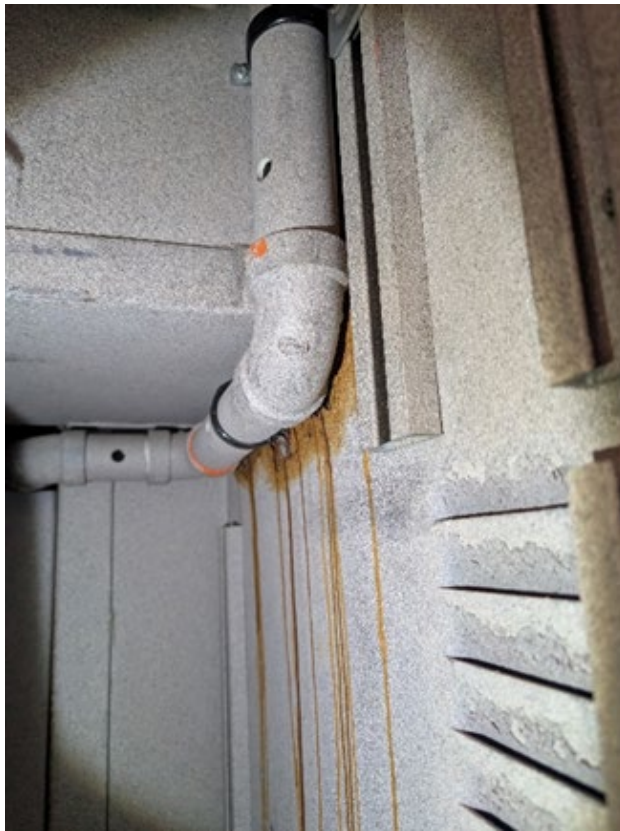
A water leak in the rear compartment near the compartment tear.
