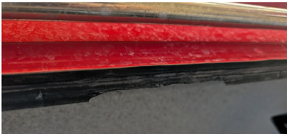
Replace defective gasket on the rollup doors.
