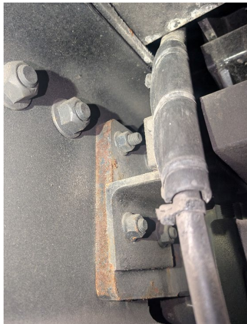
Rust was noted on the underside of the apparatus, which needs to be mitigated.
