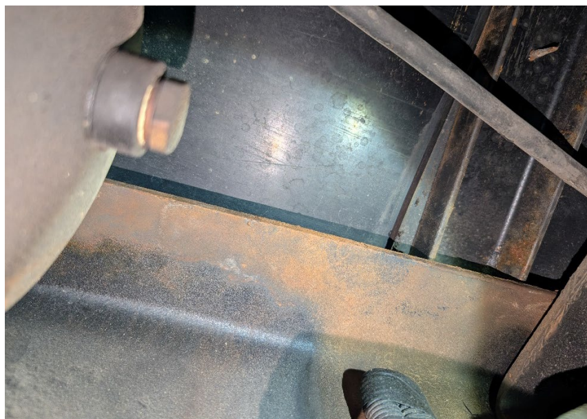
Rust forming on the apparatus sub frame and surface rust on the frame rail.
