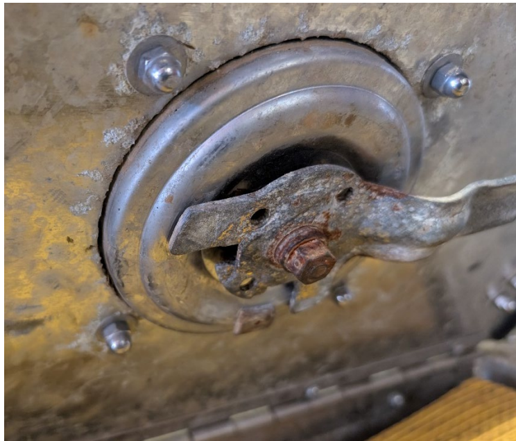
More rust and corrosion, which is not normally seen on a 2020 apparatus.
