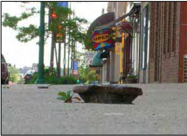
Exhibit 5-31: The curb box protrudes into the walking area after frost heaving, creating a tripping hazard.
