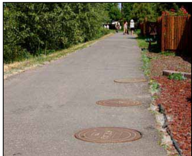
Exhibit 5-30: Where maintenance features are located in the walking area of a sidewalk or path, they must be flush and level.
